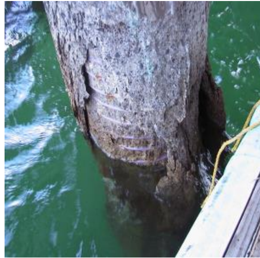
Contamination and chemical degradation problems
