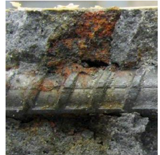
Corrosion initiation + propagation problems
